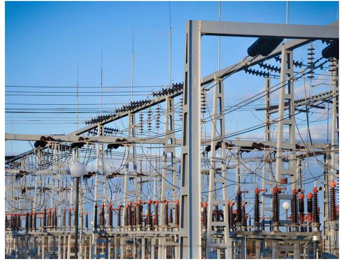
An above-grade transmission substation infrastructure.
